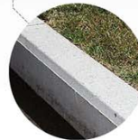
Precast Concrete curbing
