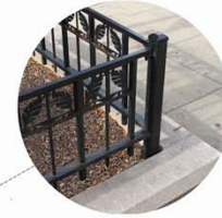
Planter rail mounted within plant bed
