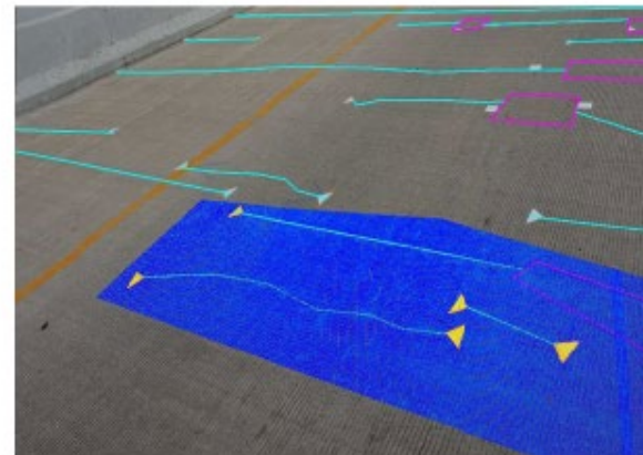
IMAGE, SCAN DATA, AND DRAFTED 3D LINES OF CRACKS
